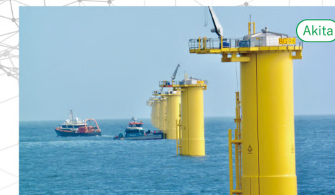
Offshore wind power generation in Akita
