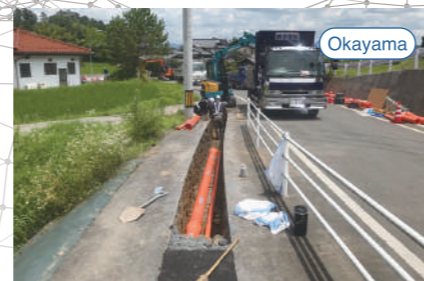
Mimasaka solar power generation plant self-managed transmission line
