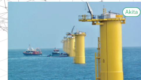
Offshore wind power generation in Akita
